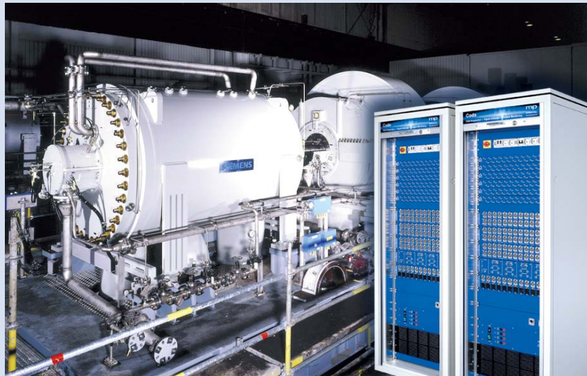
Turbomachinery test facility at Siemens, Duisburg/Germany
